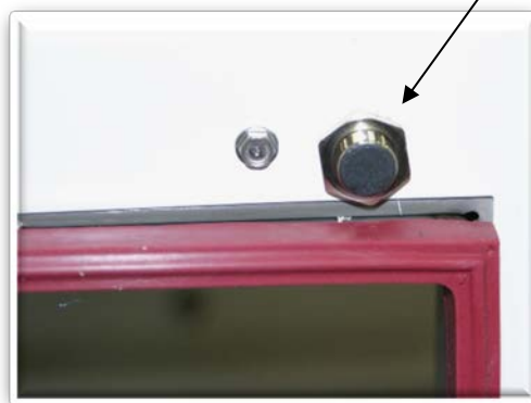
Figure 14: Airlock Door Sensor
